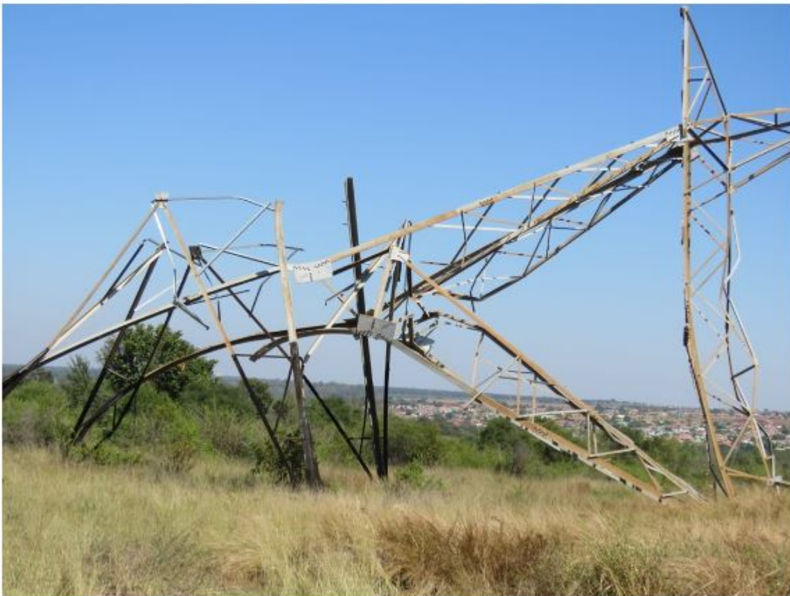
A collapsed Eskom pylon in Hammanskraal. Photo: Eskom
