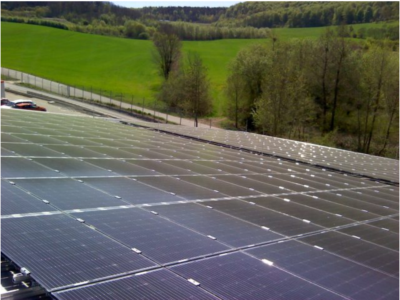
Photovoltaikdach, eigenes Werk Ute Bergner
