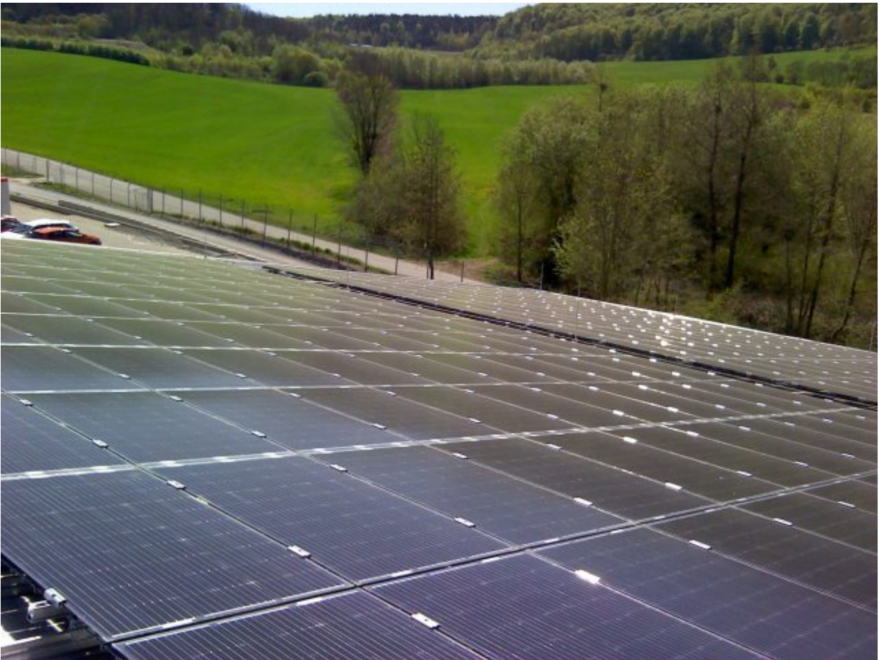
Photovoltaikdach, eigenes Werk Ute Bergner
